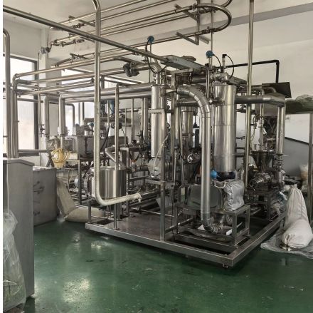
Supplier reference: real industrial steam spice-treatment equipment with process piping and controls.
