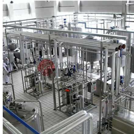
Supplier reference: real hygienic tank, piping and heat-treatment installation used for controlled liquid-food fermentation.
