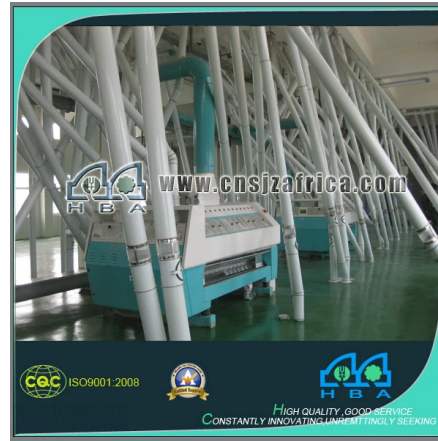
Supplier reference: installed roller-milling and conveying equipment used in barley-flour production plants.
