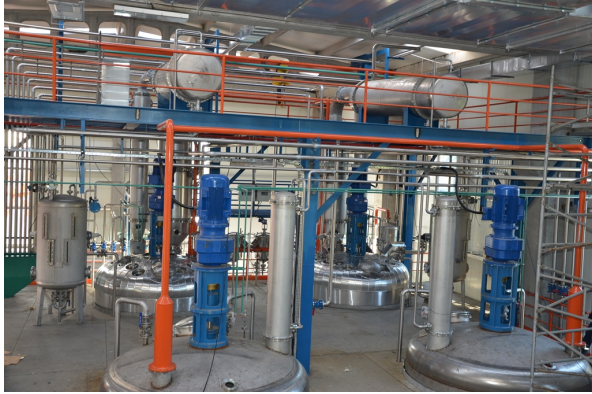
Real industrial chemical-process installation used as a reference for the contained reaction and transfer scope; final PFS equipment must come from the licensed process provider.
